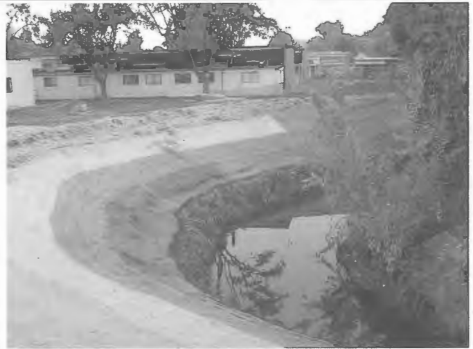
Alhambra Creek at Martinez Adult Education Restoration Project, after construction and with its newly planted willow stakes and native seed mix already blossoming.
